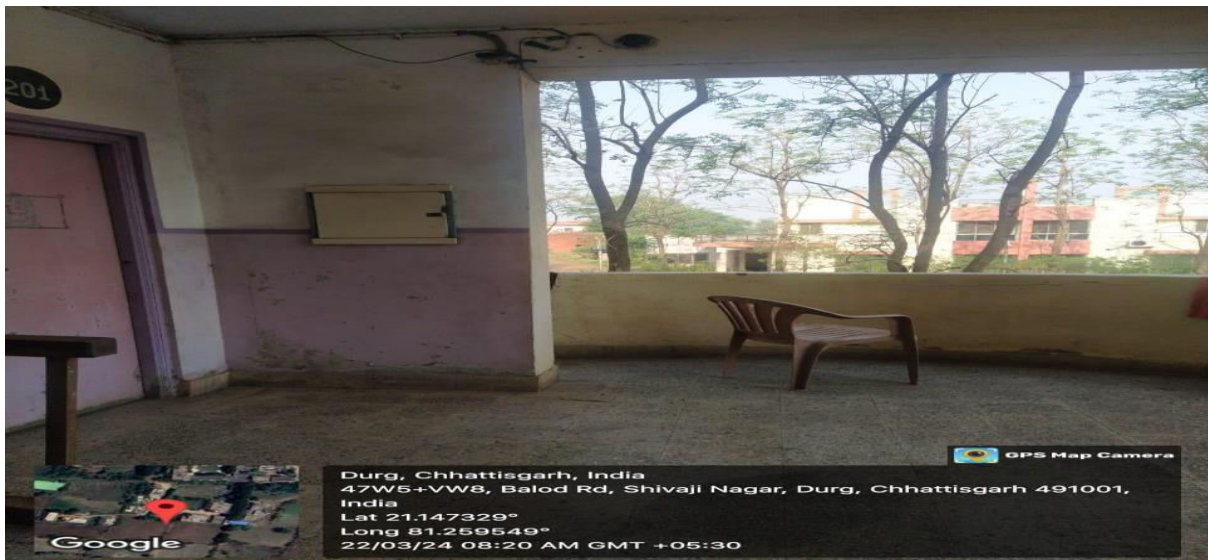
CCTV Camera Installed at Girl's Hostel
