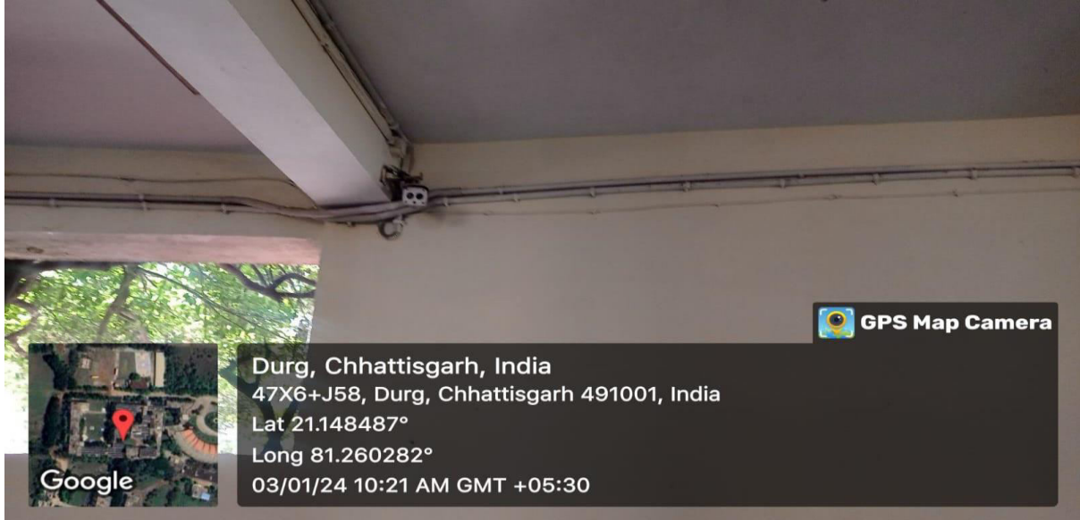
CCTV Camera Installed at College Campus
